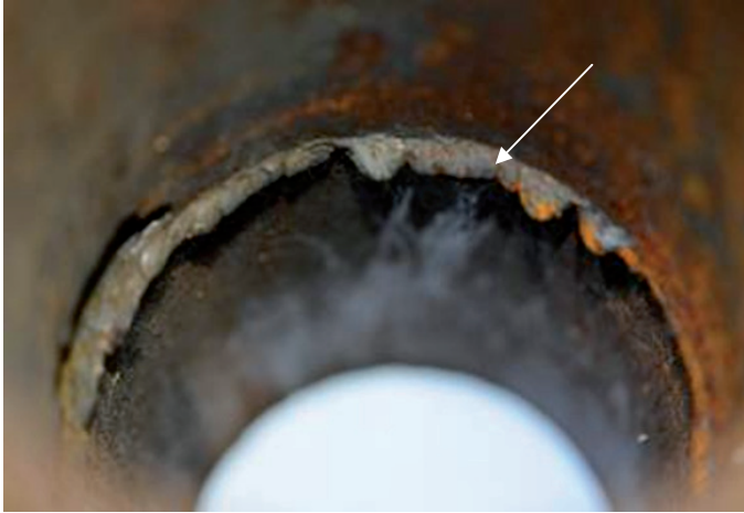
Figure 14. The inner side of circle area in Fig. 11 showing an excessive overfill (arrow) in the failed pipe at 12 o'clock position.
