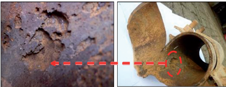
Figure 8. Wall thinning and pits at 5 – 7 o'clock position of upstream part.
