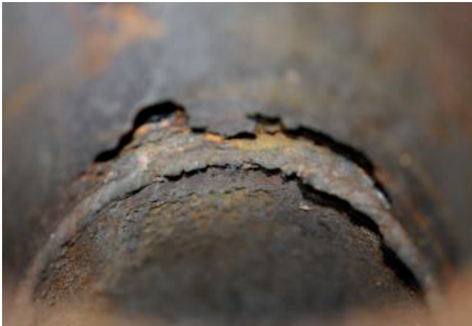
Figure 15. An excessive overfill and severe surface degradation beside overfill at 6 o'clock position.
